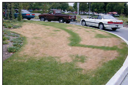
Figure 4 - Misplaced sprinklers and trenches not properly compacted.
