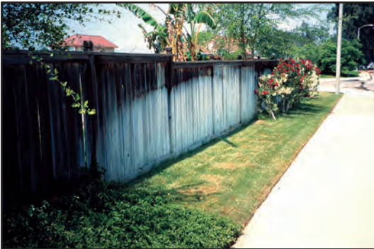
Figure 5 - Wood fence bleached by sprinkler spray.
