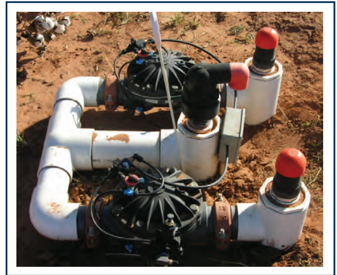
FIGURE 3. Example of a field installation of pressure regulating valves and air release vents
