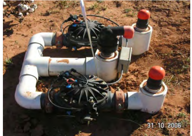
Figure 2.3. An example of a field installation of pressure regulating and air release valves.
