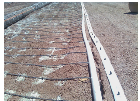
FlatNet laid out with threaded fittings inserted prior to drip laterals being connected and FlatNet with drip laterals connected and at operating pressure.
