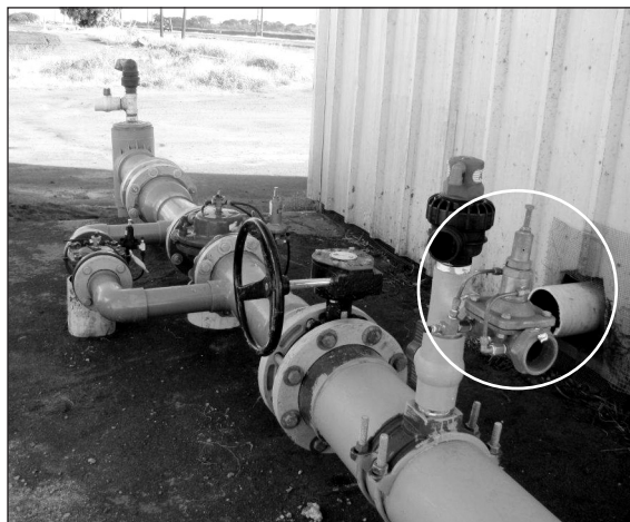
QR Valve located upstream of a sand media filter.
