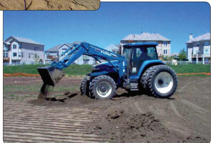
Figure 20 - Mechanized Equipment May be used to spread soil over the top in larger systems. It is important to evenly spread the soil moving with the tubing direction to keep the laterals from shifting.
