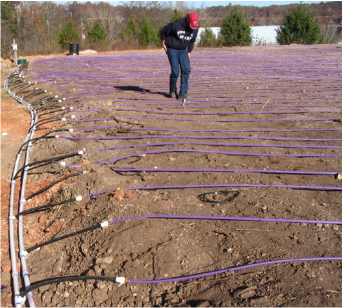
In order to establish an adequate soil base for the field, over 18" of fill was brought in. Notice the use of flex PVC to transition from the supply and return headers up to the dripperline laterals. This helps to protect the dripperline from damage in poor soils as well as preventing drippers from being placed outside the boundary of the drip field.
