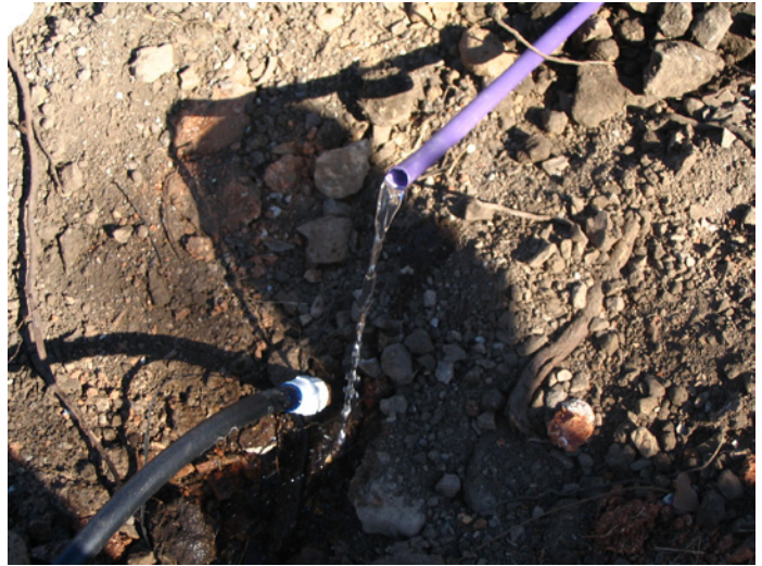
Fresh water was used to purge any construction debris from the Bioline before attaching it to headers. This also provided an excellent visual confirmation that there were no damaged laterals before cover soil was added.
