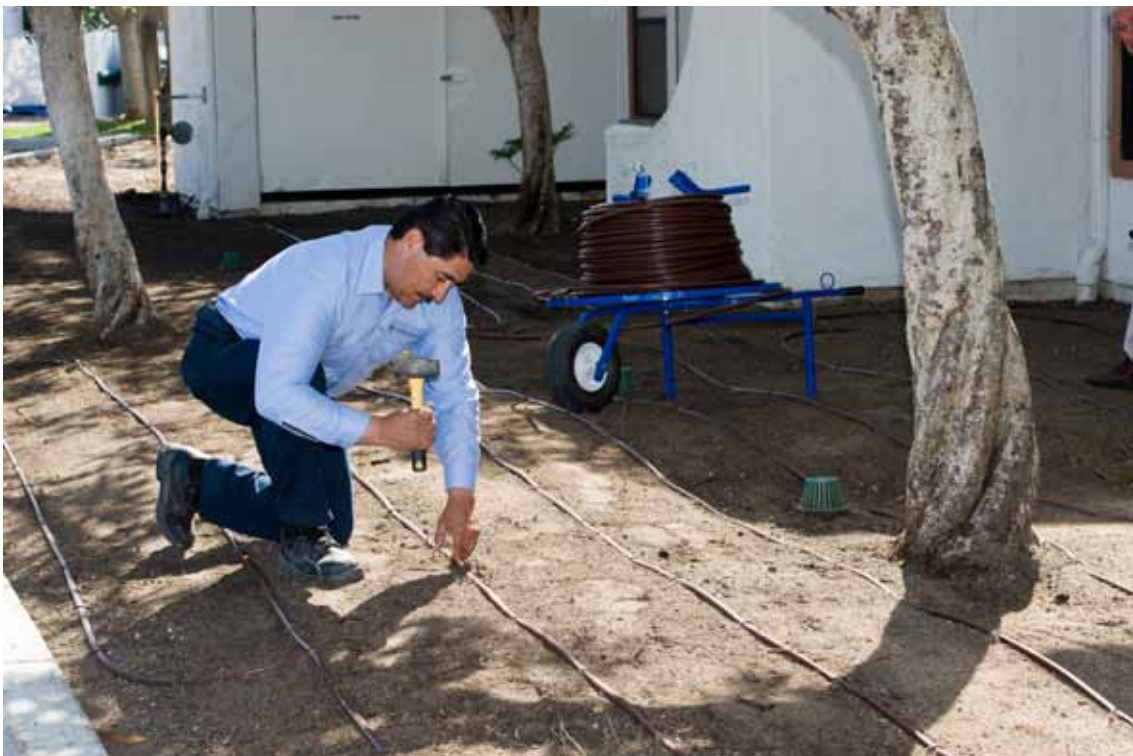
Joe Chavez, Viridian crew member, installs over 20 miles of Techline CV in more than 10 acres of landscaping, covering each planted hydrozone.
